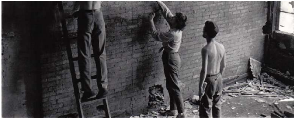
Renovations at 498 Broome Street, New York, ca. 1963 from the Soho Memory Project
